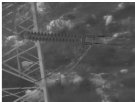
图 11 故障跳线联板识别结果 Fig.11 Fault jumper connecting plate recognition result
